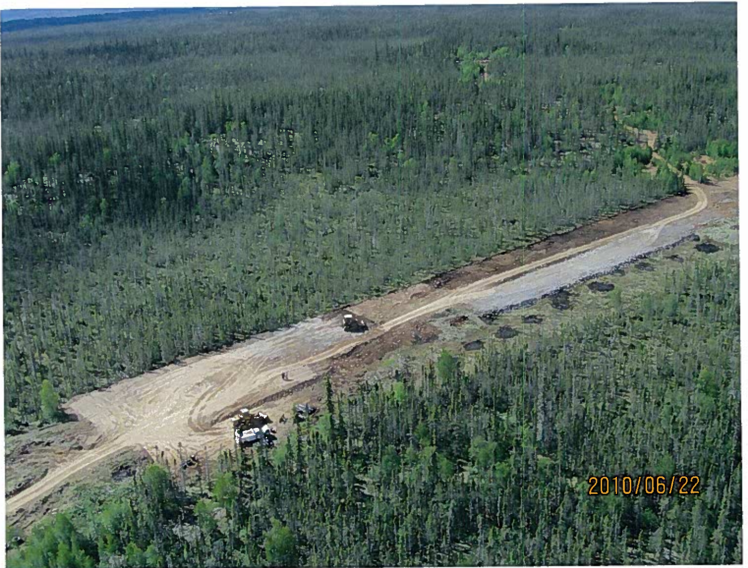
MV2010G0001 - Avalon Rare Metals Inc. - Thor Lake Looking southwest at the airstrip being constructed West of Thor Lake.
