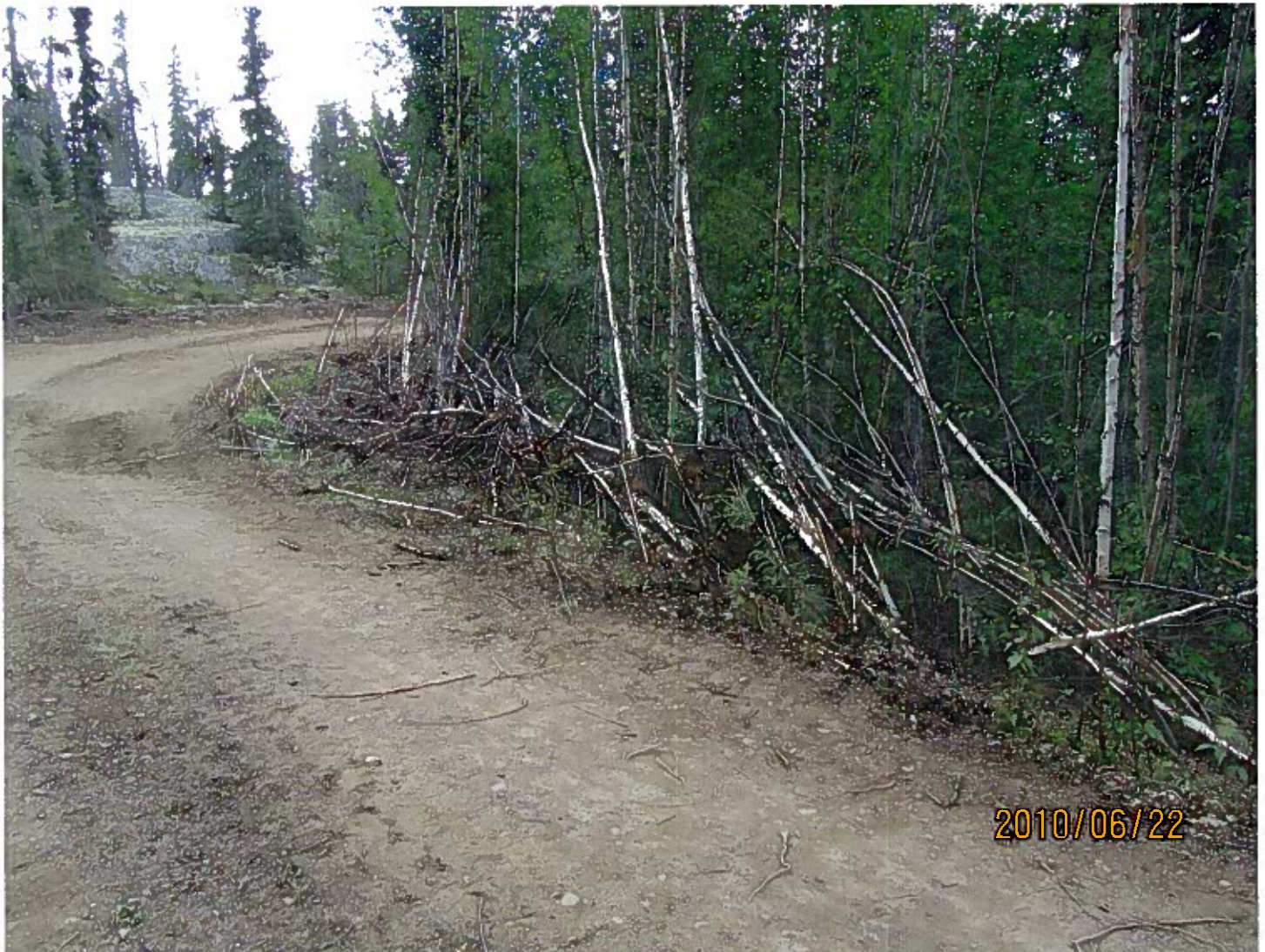
MV2010G0001 - Avalon Rare Metals Inc. - Thor Lake Vairous areas along the road system that have leaners present that must be disposed of as per the permit operating conditions.
