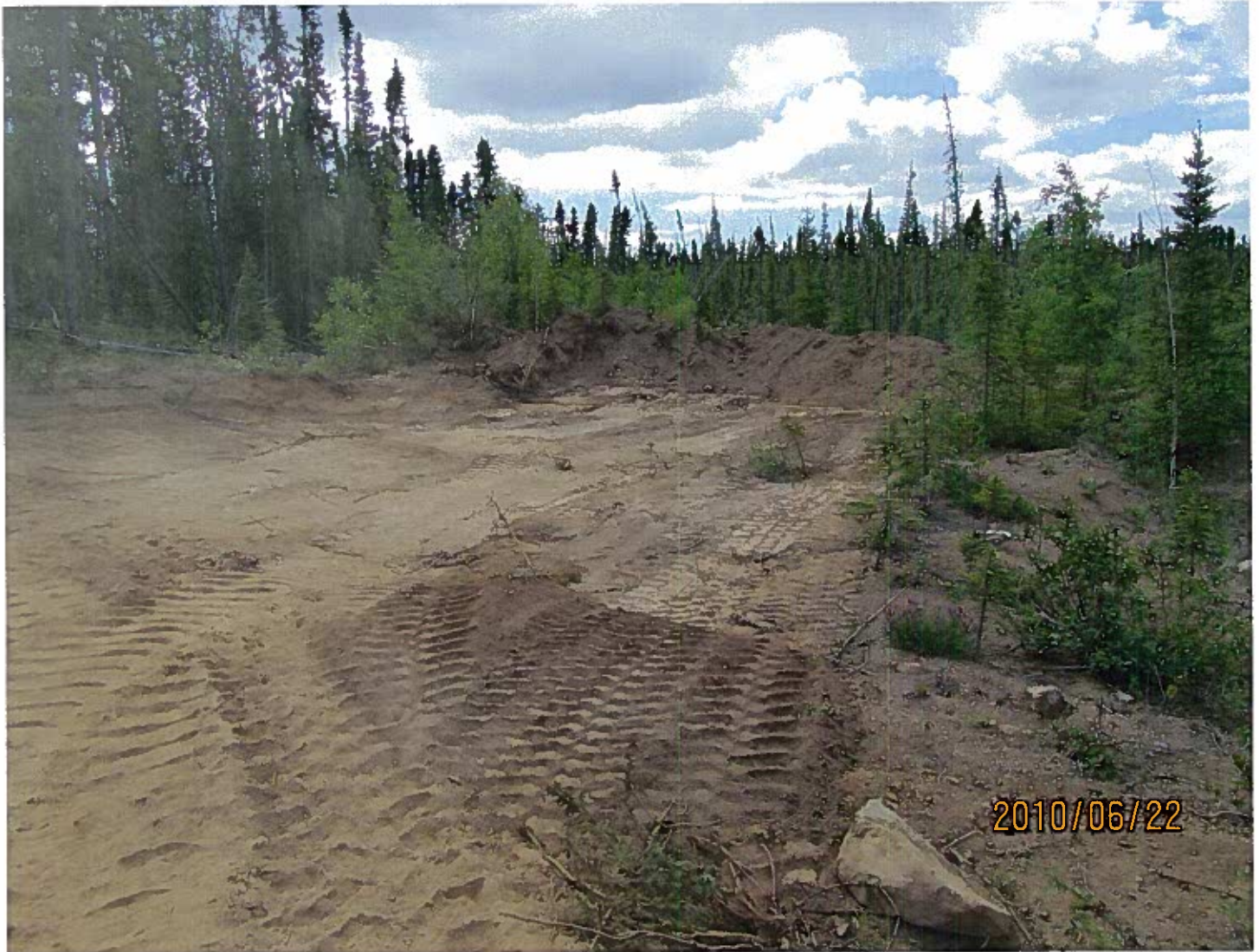
MV2010G0001 - Avalon Rare Metals Inc. - Thor Lake Push out along the all weather road that must be pulled back and re-contoured.
