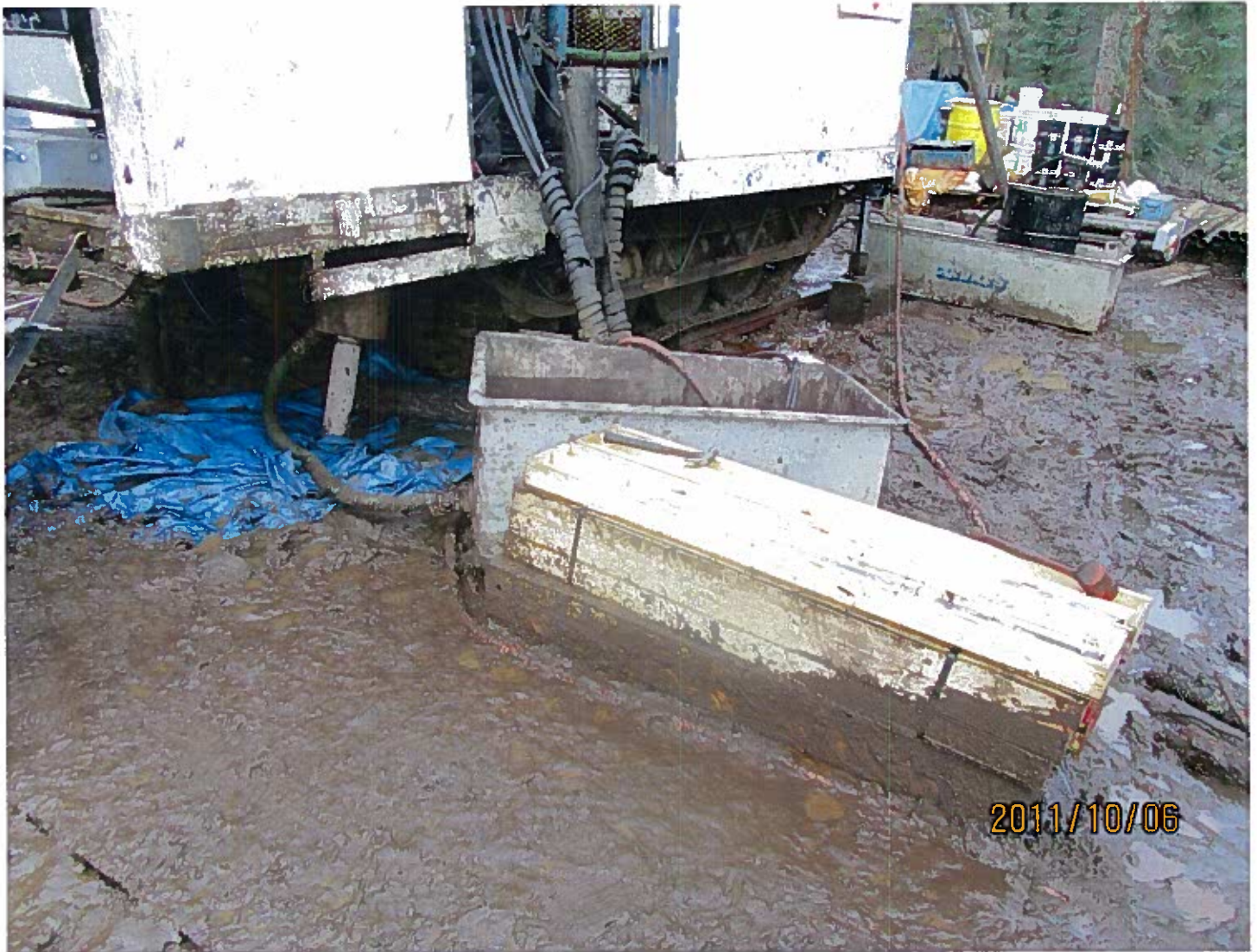
Photo #5 - Avalon Rare Metals Inc. - Thor Lake Tub at the buggy drill for the collection of drill water and cuttings to assist with proper water management.
