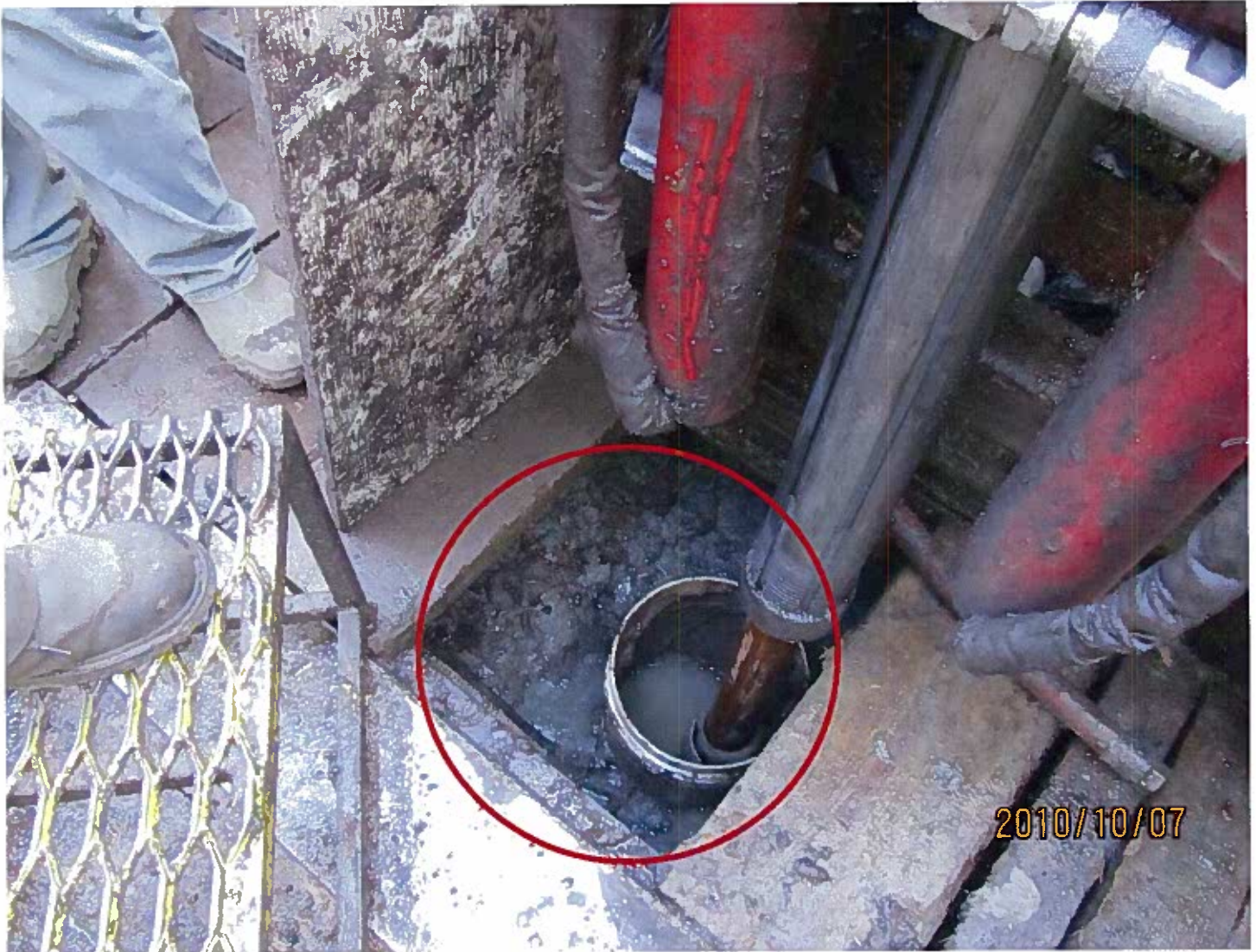
Photo #3 - A sump has been excavated below the casing at the skid mounted drill to collect drill cuttings and water to allow for proper disposal away from the drill pad.
