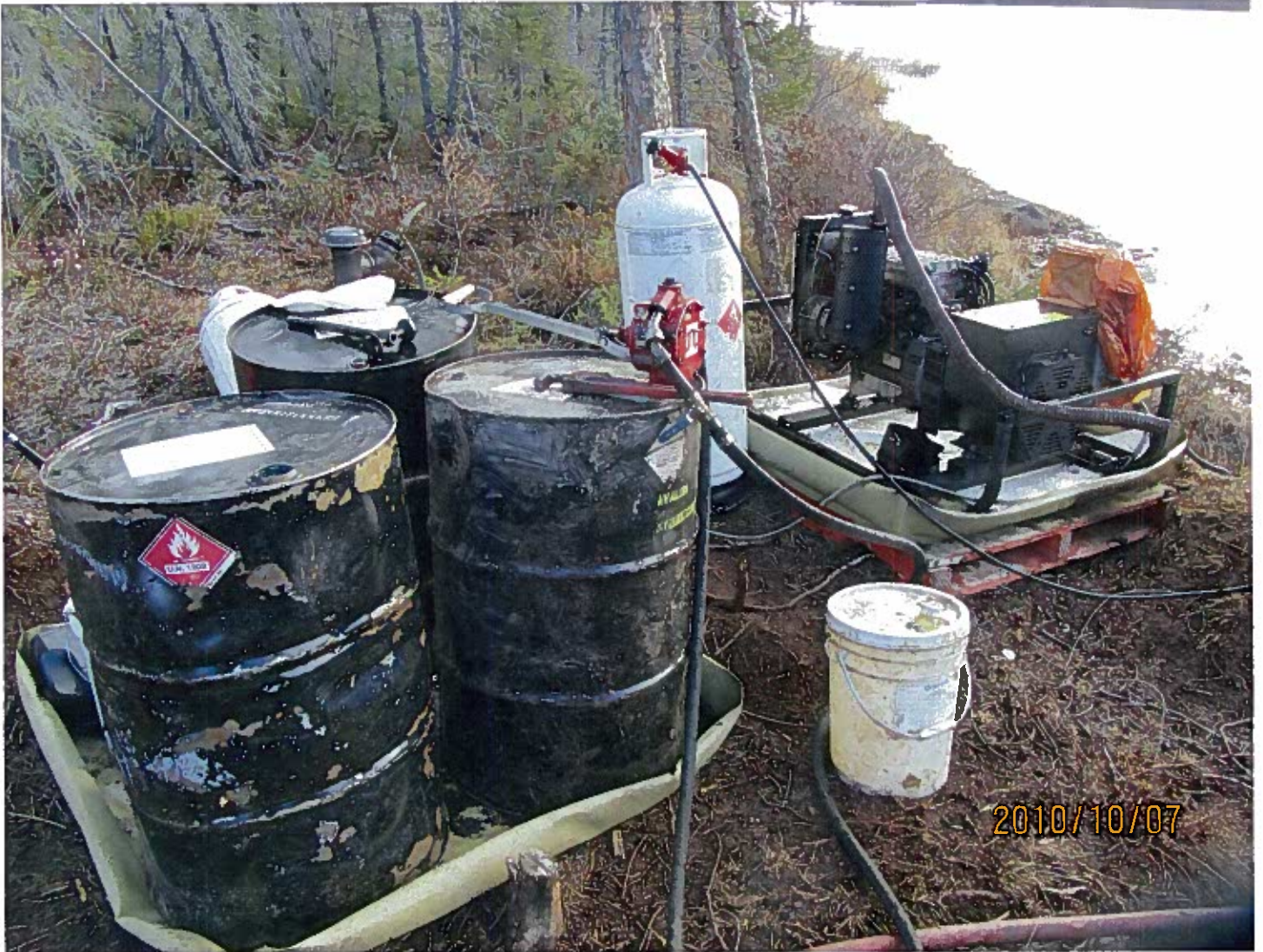
Photo #7 - Water pump and associated fuel by the shoreline of Long Lake. Secondary containment below the fuel drums and water pump was satisfactory, but the Permittee must ensure that they are maintained to prevent them from filling up with water and over topping.
