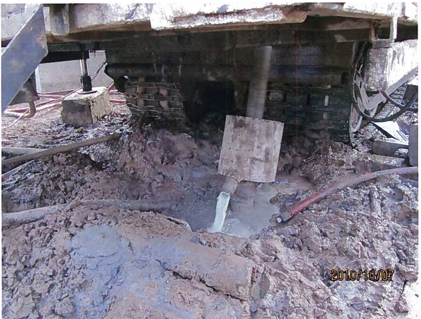
Photo #6 - Sump to collect drill water and cuttings has been excavated below the casing on the buggy drill. Proper disposal is occurring at this drill.
