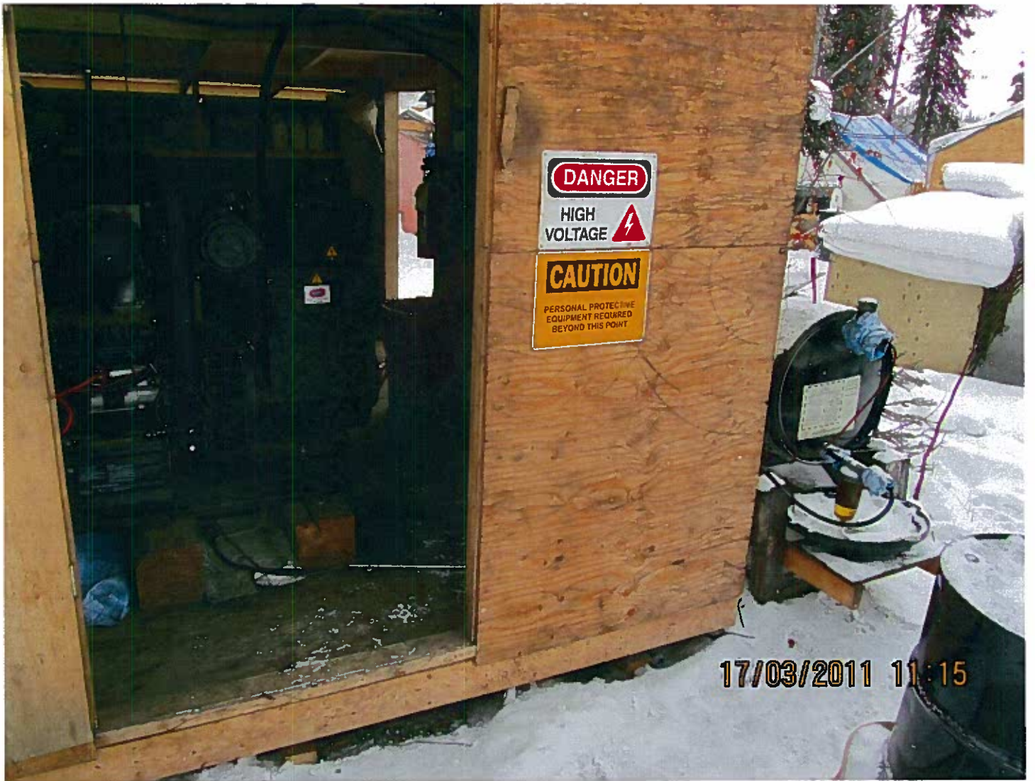
MV2007C0039 - Avalon Rare Metals Inc. - Mineral Exploration - Thor Lake, NT. Generator at the camp has been lined with absorbents to capture potential leaks or drips.
