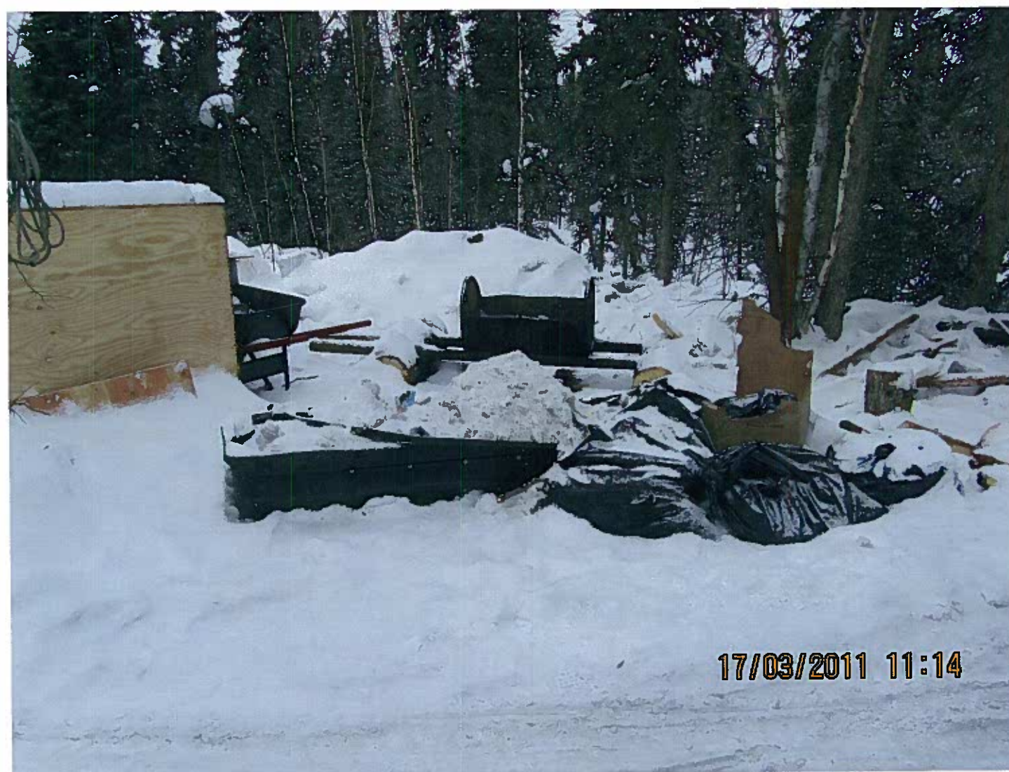
MV2007C0039 - Avalon Rare Metals Inc. - Mineral Exploration - Thor Lake, NT. Hydrocarbon impacted snow and ice from minor spills is being collected, thawed and treated on site.
