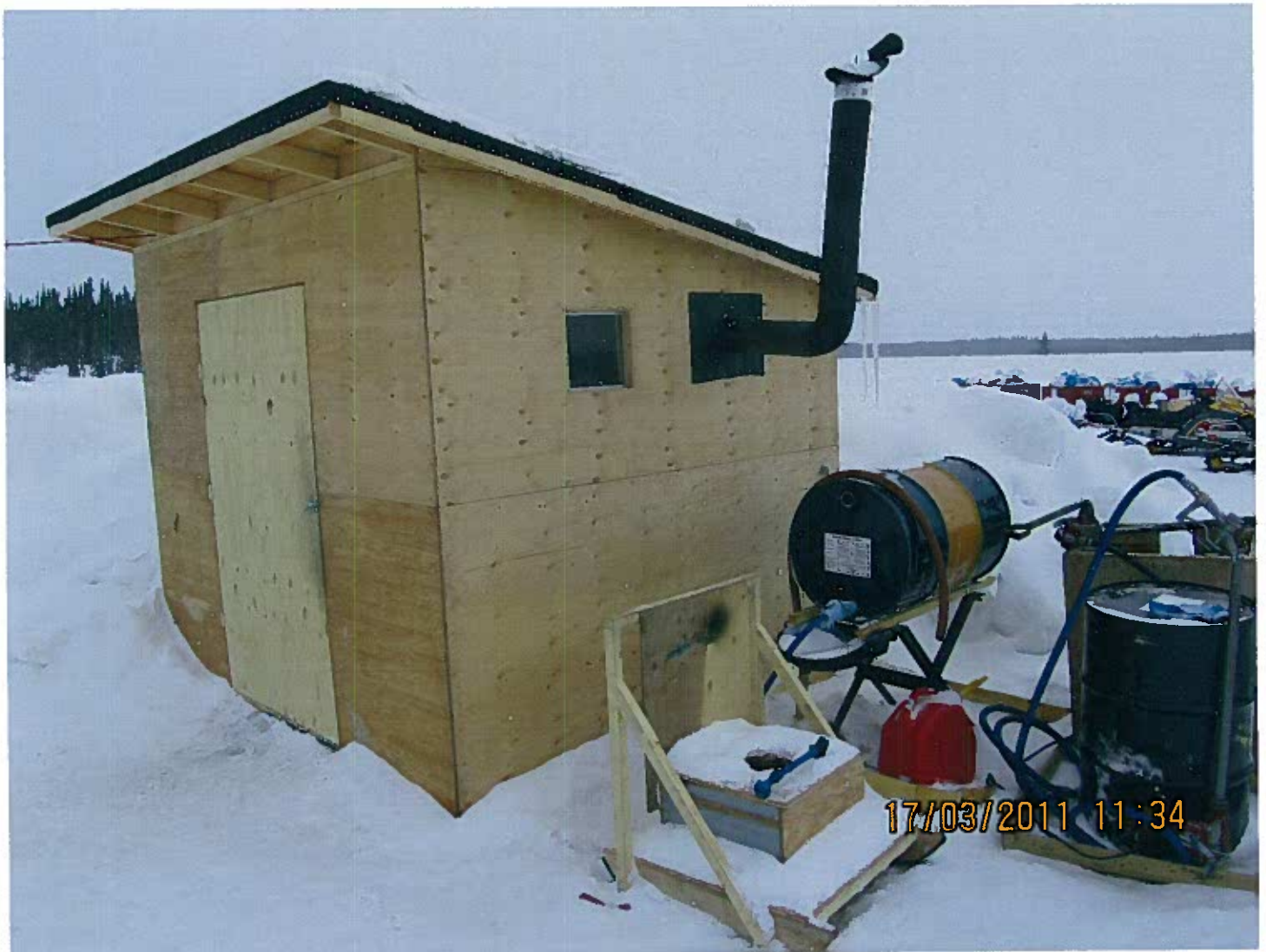
MV2007C0039 - Avalon Rare Metals Inc. - Mineral Exploration - Thor Lake, NT. Pump shack has been constructed to house water pumps and hoses. Fuel for the shack is within secondary containment.
